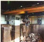
Fully automatic Munck crane in operation in an incinerator plant in Oslo Norway.
