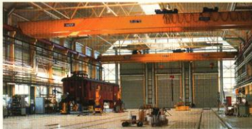
Duo industrial cranes installed at NSB-Norway
