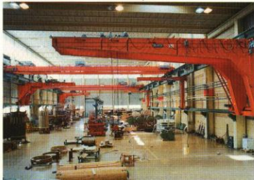
Wall mounted cranes at ABB, Drammen-Norway
